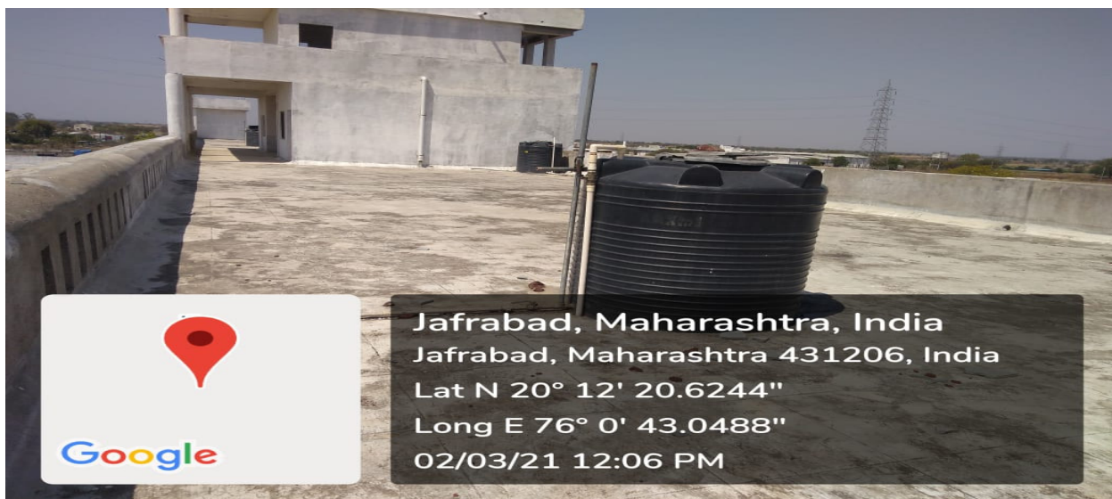
Water distribution system of the college
